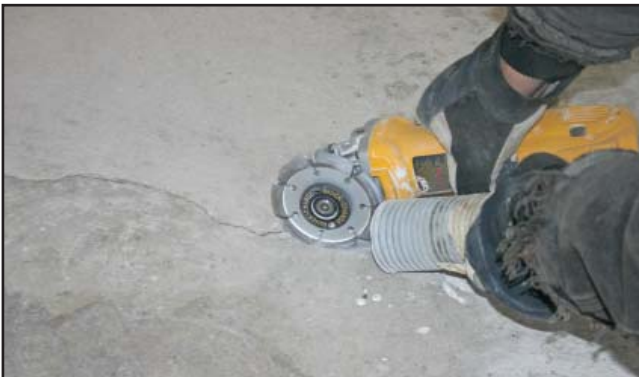
Opening the Crack
